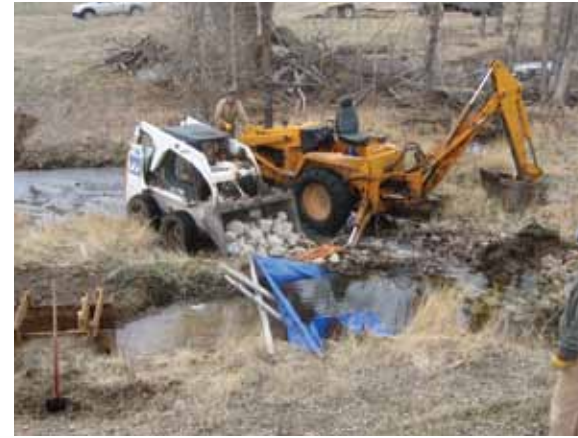
Dry Cottonwood Creek Ranch used a portion of their water leasing payment for upgrading their irrigation diversion dam and headgate.
