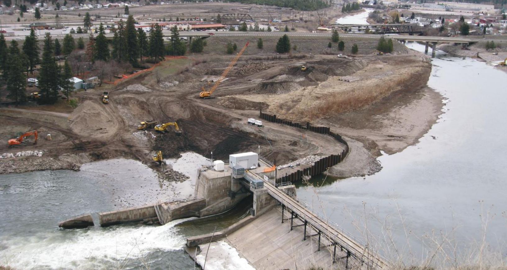
Dam removal underway: powerhouse removed; spillway still in place. Blackfoot River enters from top right.
