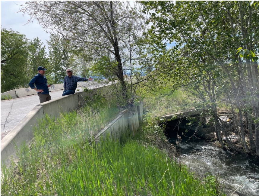
Grant Creek flowing through an under-sized culvert
